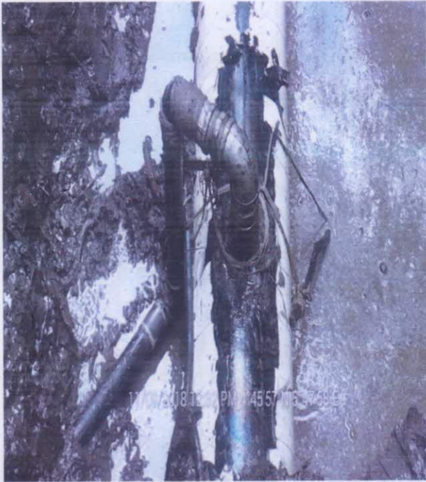
2"VALVE AND PIPE LEADING TO THE CAMP.
